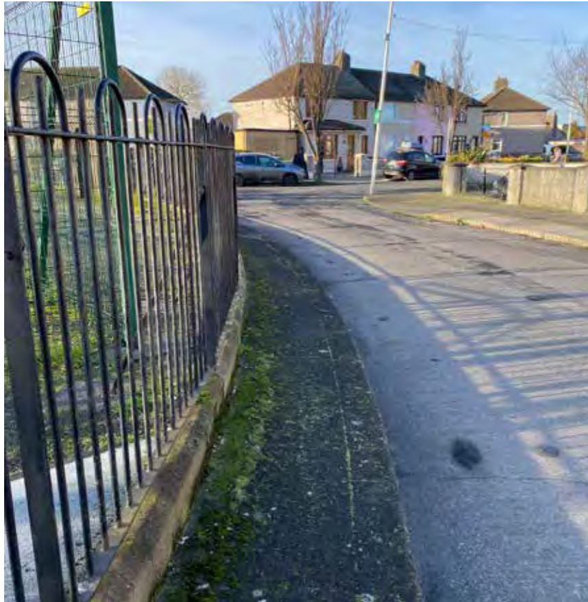
Existing footpath (c. 800mm wide) and railings and pitch fencing in background.
