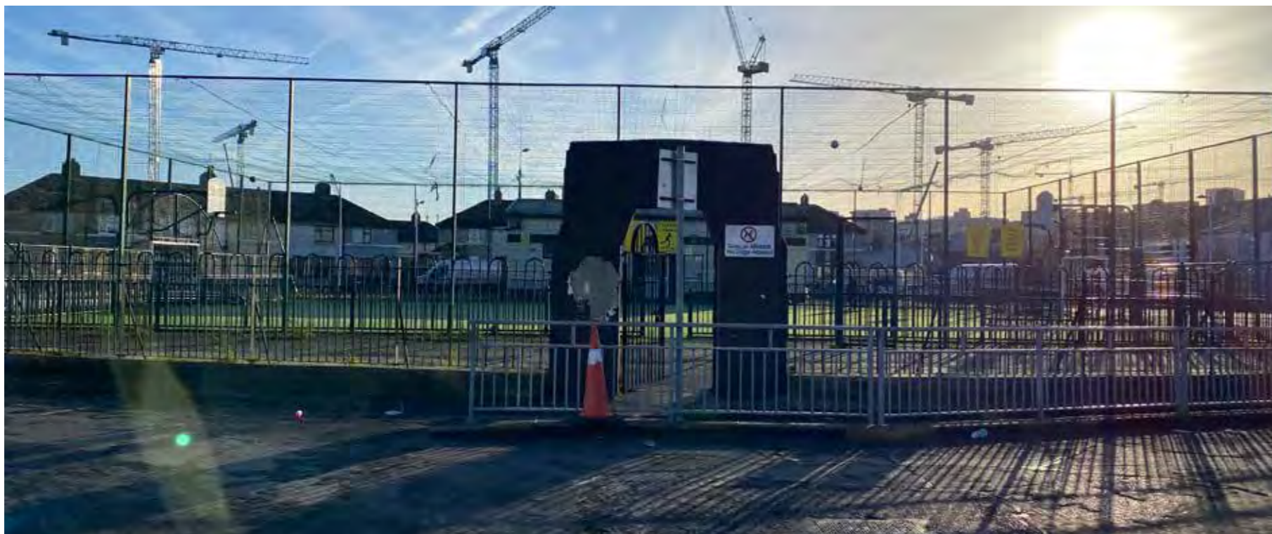
Entrance near Church Road - attempt to address safety issues onto a busy road with the installation of additional barriers - adding to general clutter of the space
